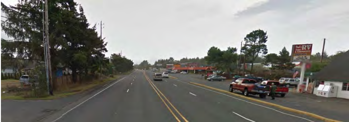
Figure 2-4 – Skinny shoulders with maintenance issues in Gerhart
